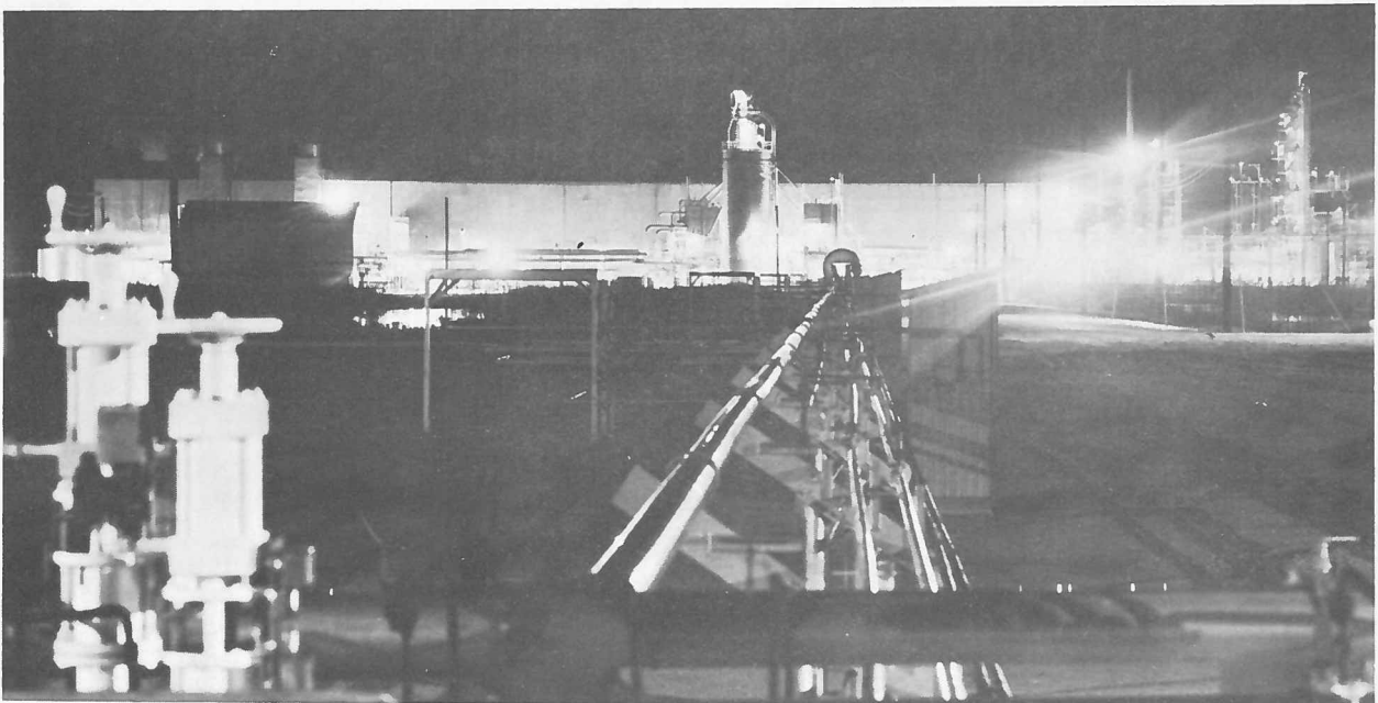
Figure 5. Vacuum-insulated transfer lines for liquid hydrogen.
