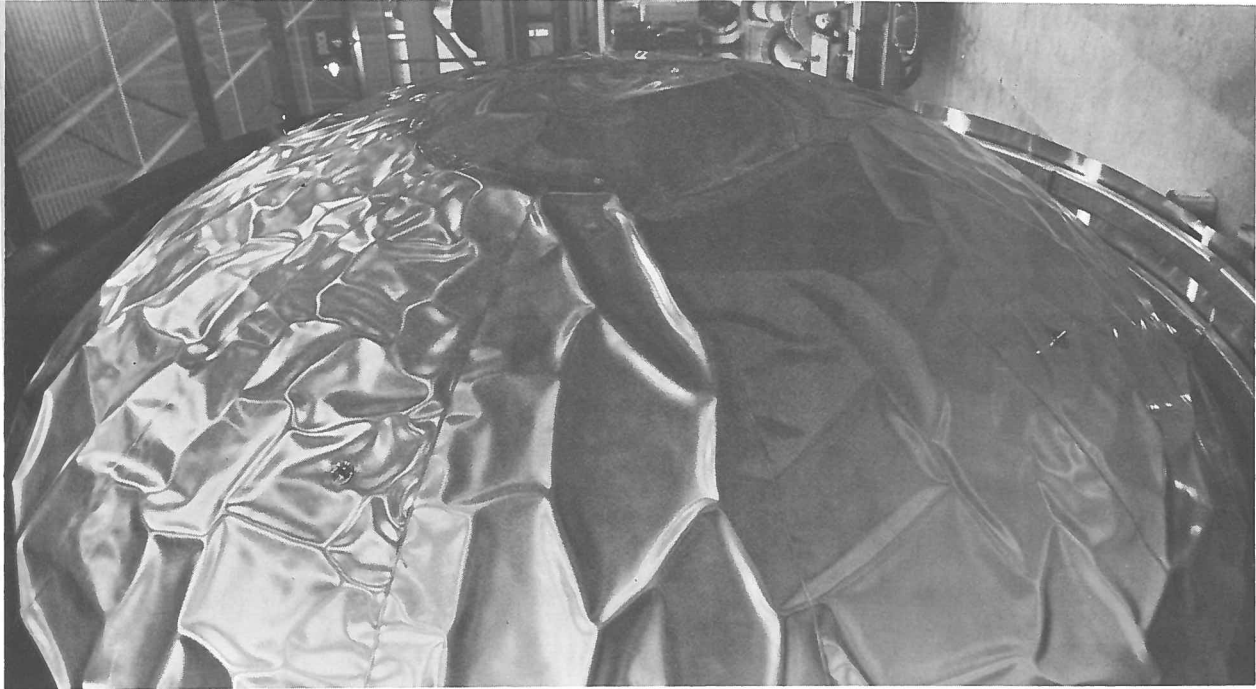
Figure 18. Wrinkled skin of vacuum insulation.
